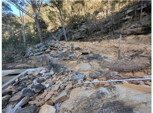
The car turnaround area next to the weir and fishway will be repaired.
